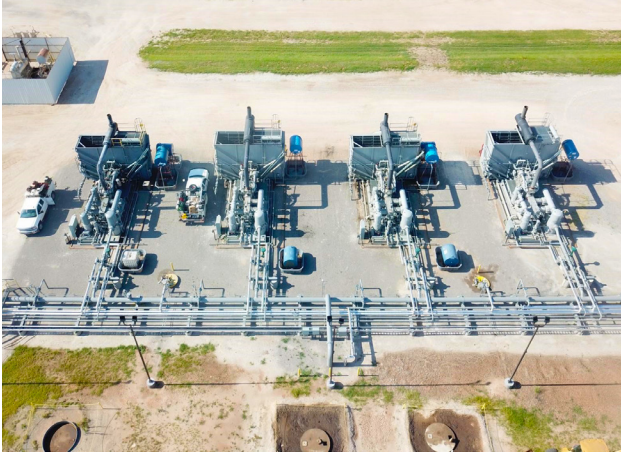
Fig. 1: Natural Gas Compressor Station Booster
