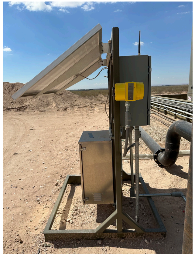
Fig. 2: Portable Flare Gas Monitoring Skid
