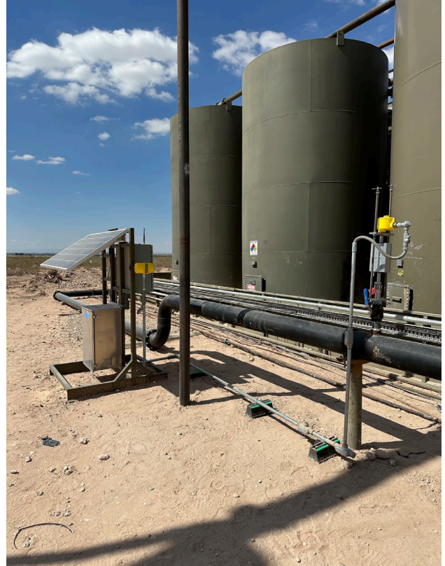
Fig 3: Portable Flare Gas Monitoring Skid - FCI ST100A
