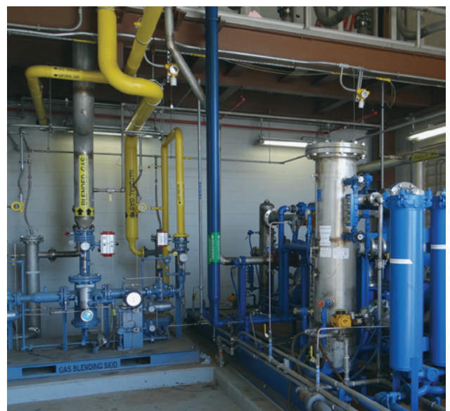
Blended waste gas and natural gas system is used to operate a New Jersey facility's co-gen engines.
