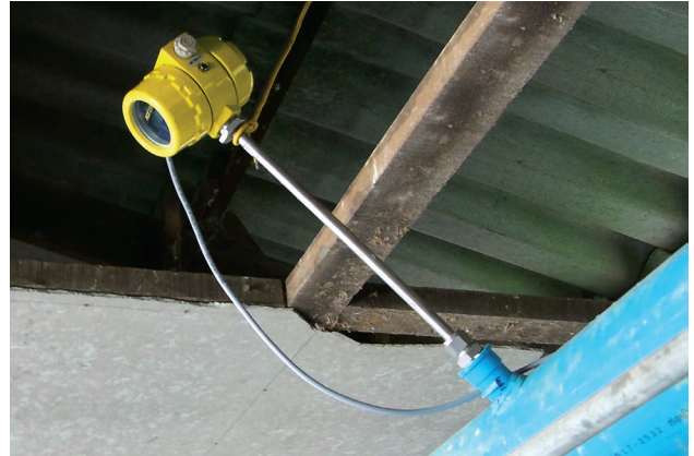
Figure 4: Flow meters installed in S.P.M. (roof interior with pipe run and meters)
