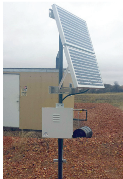
Figure 1: Solar power system at well site
