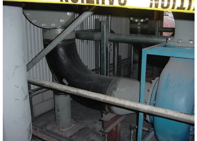
Figure 3. Electric power plant elbow and pump
