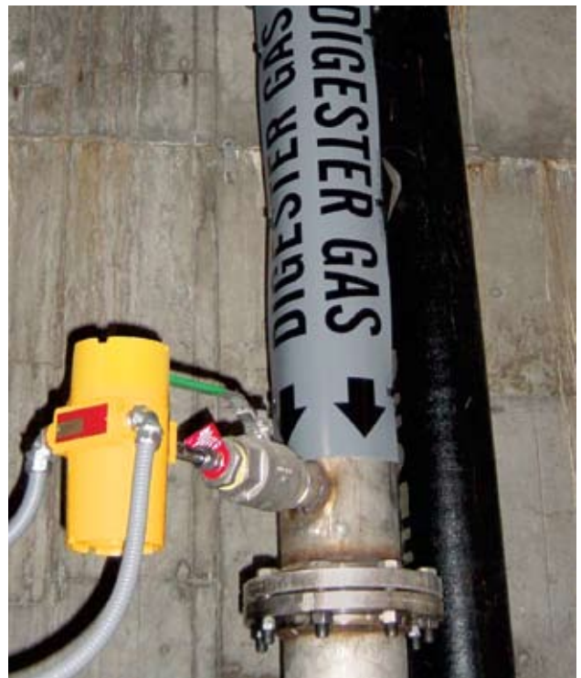
Figure 3. FCI Flow Meter installed on gas digester pipe.
