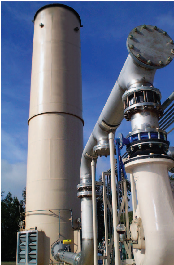
Figure 2: FCI Model ST98 mass flow meter in a landfill gas system
