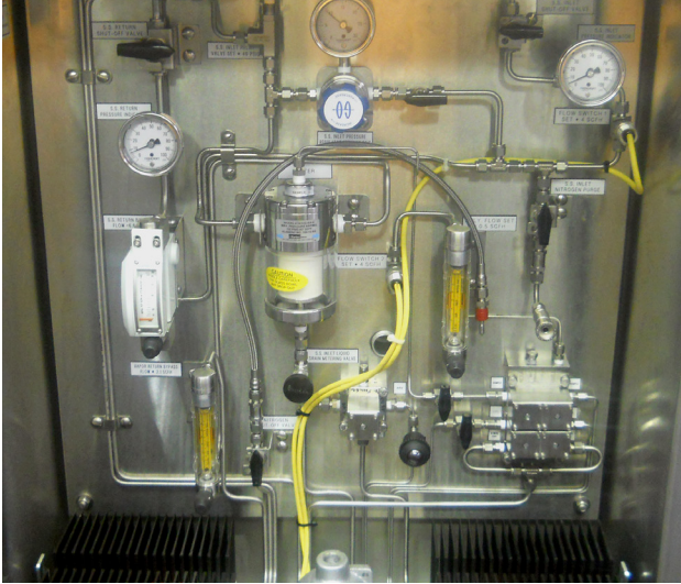
Figures 5 & 6: FS10A in remote configuration; hot process sampling system (VAM/new shelter)
